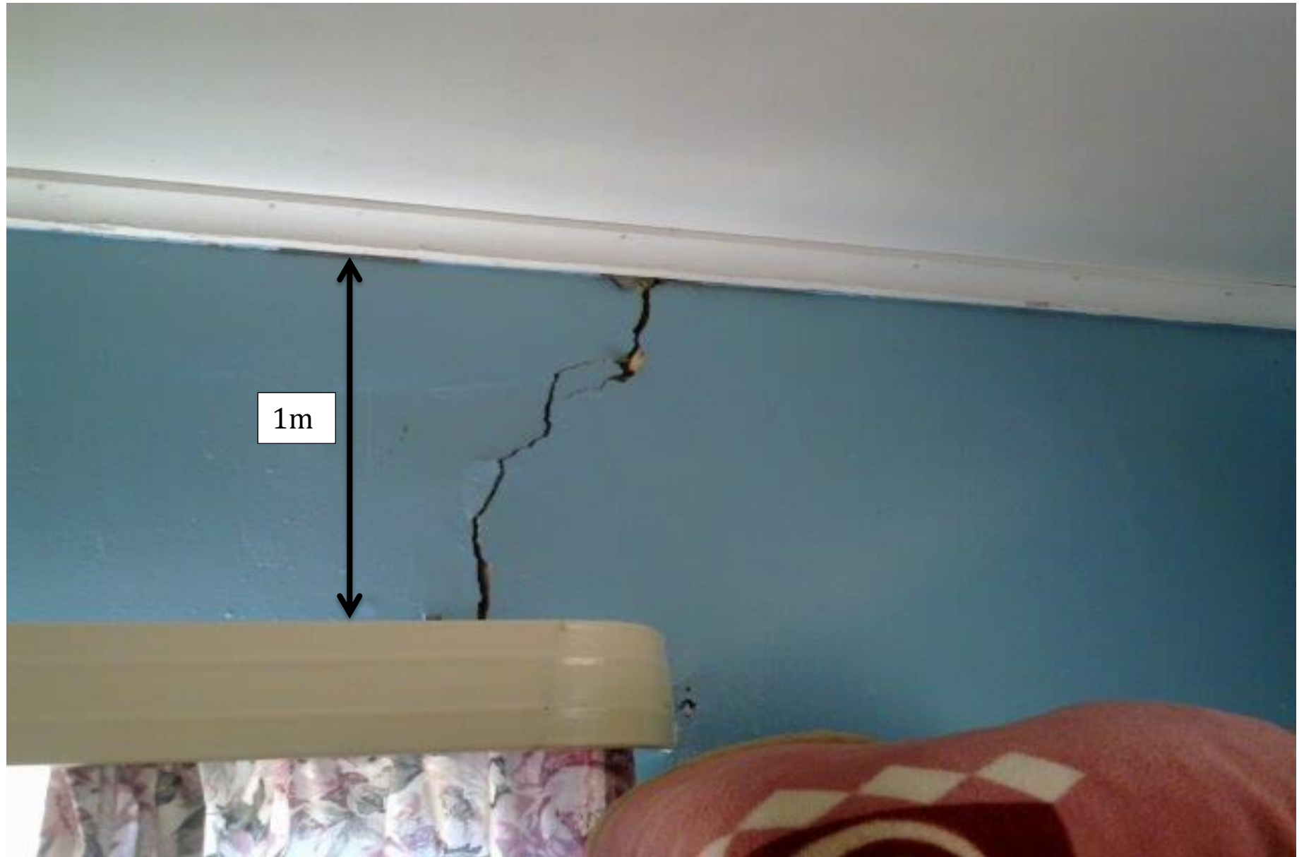
Figure 5. 21: A wall crack inside one of the Bruinhoek houses.
