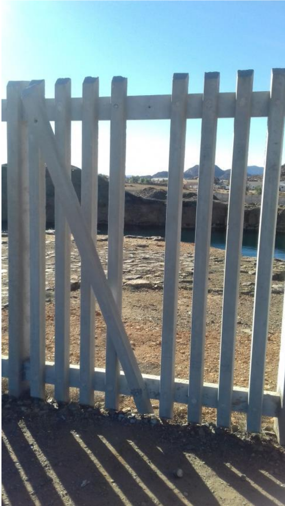
Figure 4. 6: The 2.5m high concrete palisade surrounding the West O'Okiep Mine glory hole.
