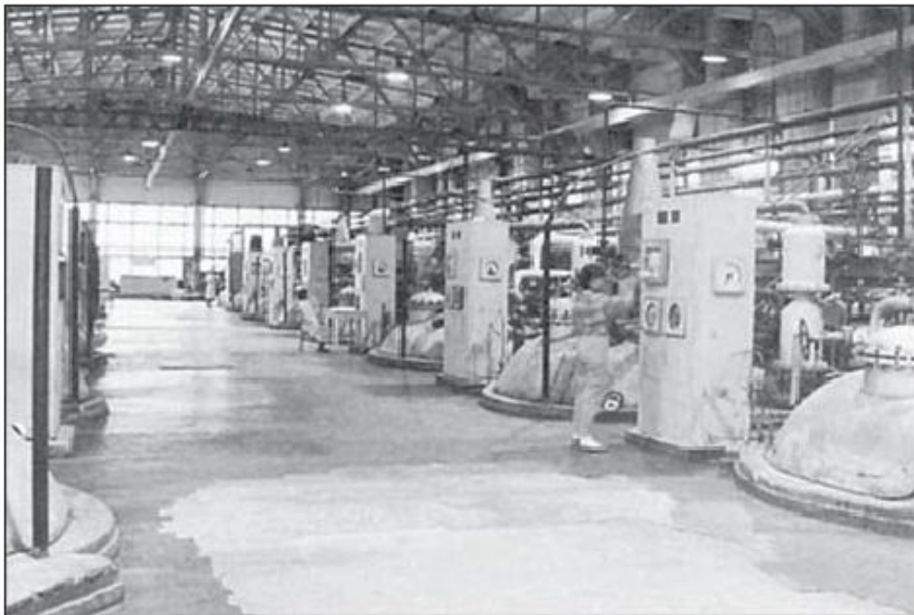
Photograph of SNOB's Building 221 interior with a row of 20,000 liter fermenters. (Photographer: Andrew C. Weber.)
