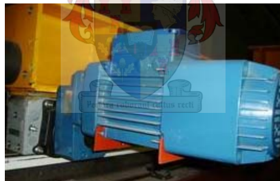
Photo 4.1: Electrical driving motor at crane wheel
