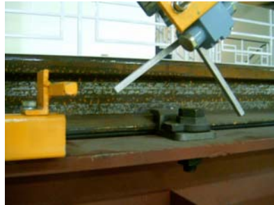
Photo 4.2: Emergency cut-out mechanism for longitudinal crane travel
