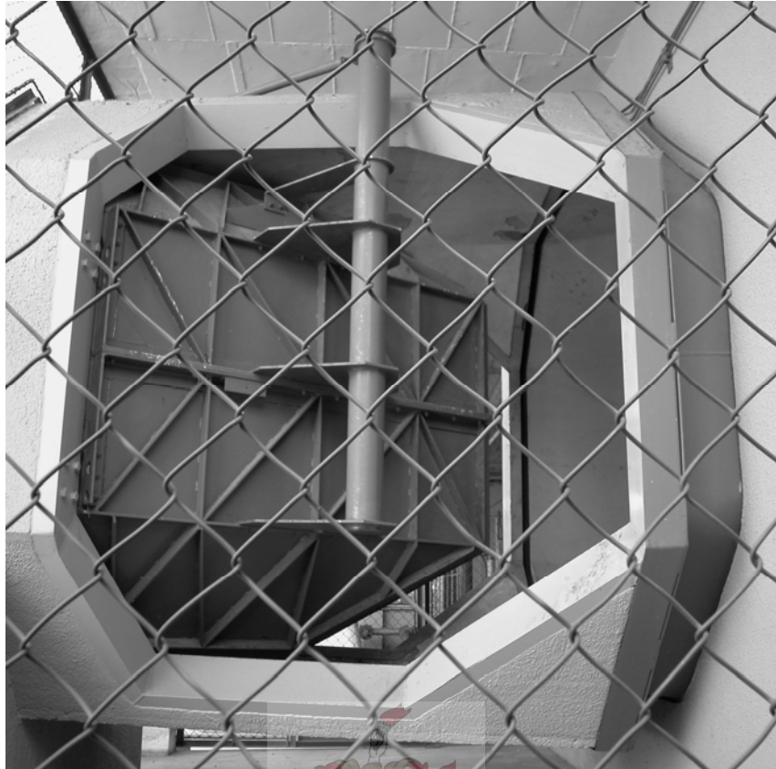
Figure 3: The hydraulic actuated doors in the closed position
