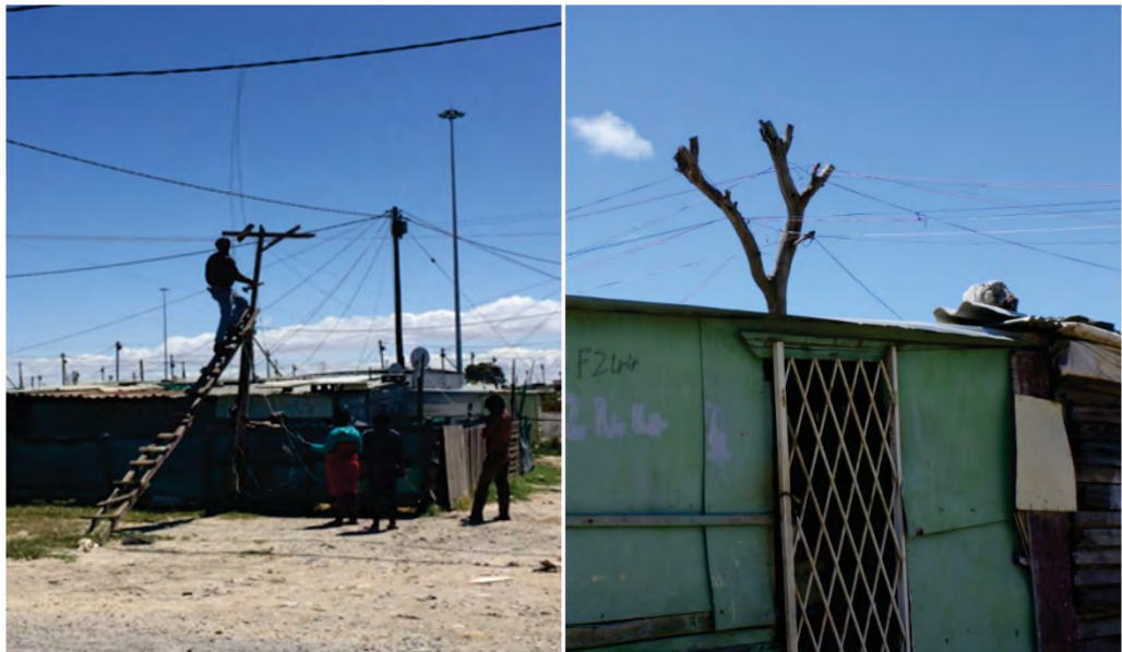
Figure 2-3: A view an informal areas showing various electrical connections that are a significant problem for fire safety
