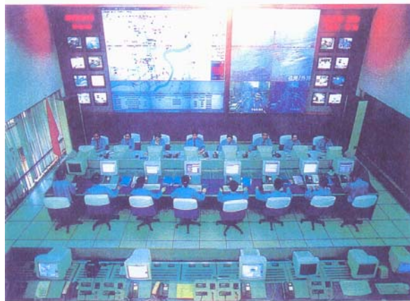
Figure 3.1 Shanghai's Control Centre
