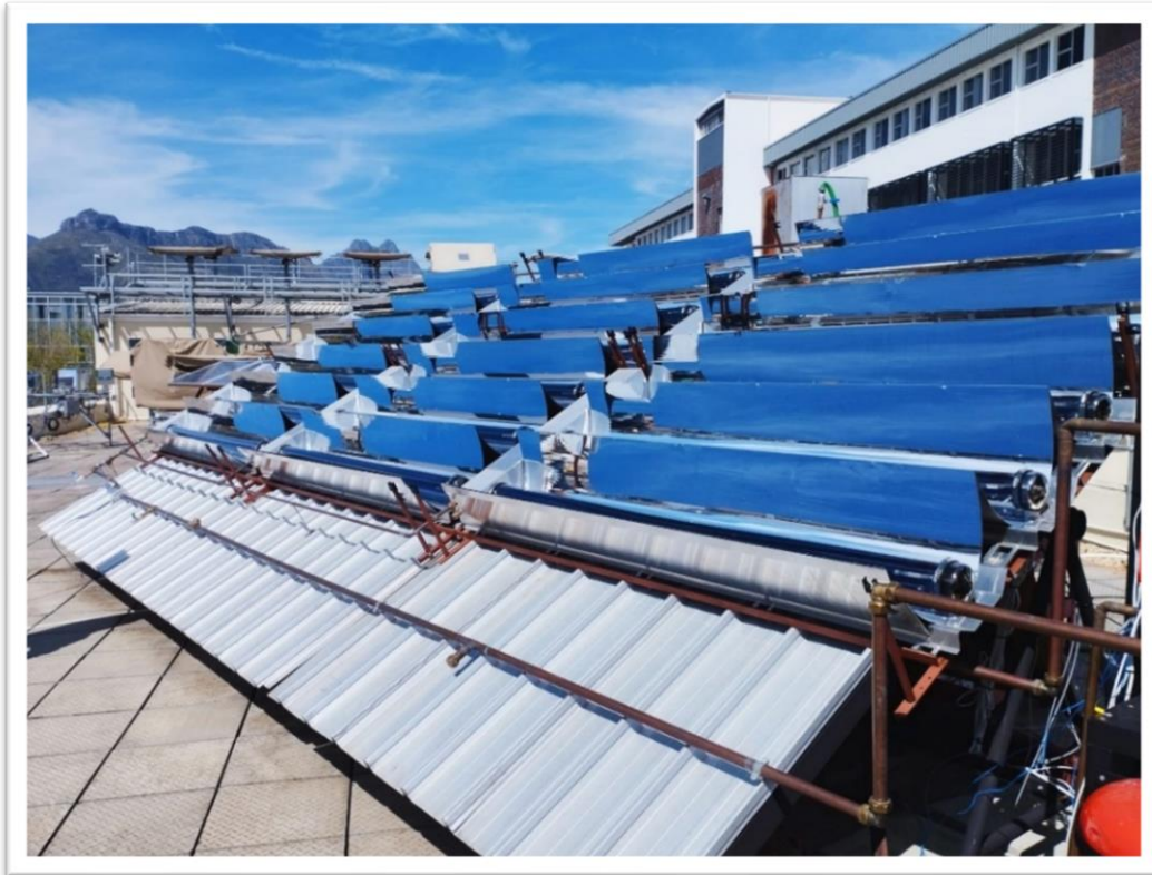
Figure 17 Solar collector array
