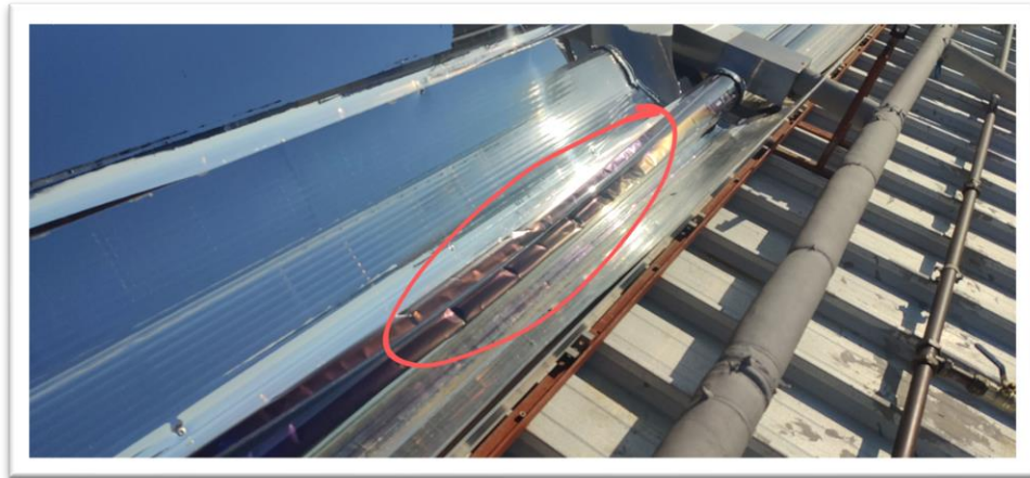
Figure 62 Copper absorber tube and fin damage around 6 months after testing
