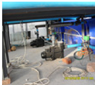
Water pumps connected to sumps & biofilter
