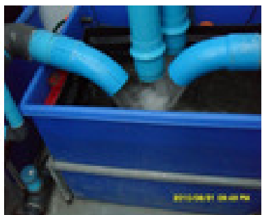
Mechanical filter connected to sumps & biofilter
