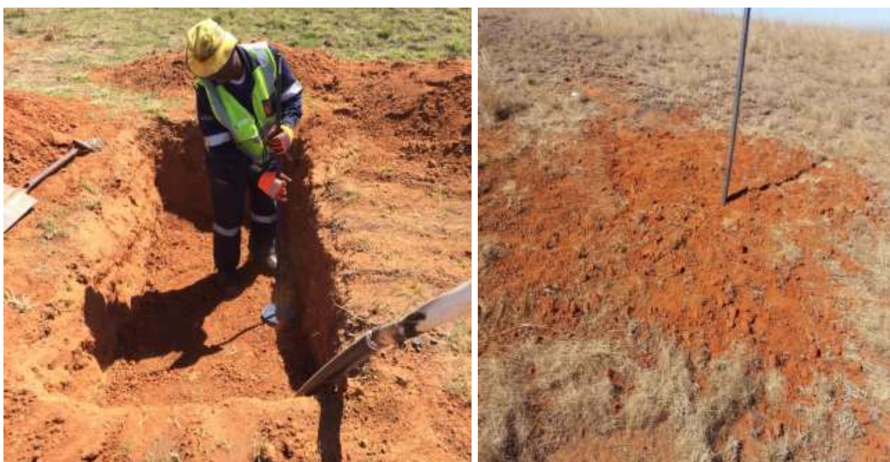
Figure 2.2: Hand compaction of 100 mm layers during pit in-filling according to cover layering on the lefthand side. On the righthand side is the surface of in-filled pit.
