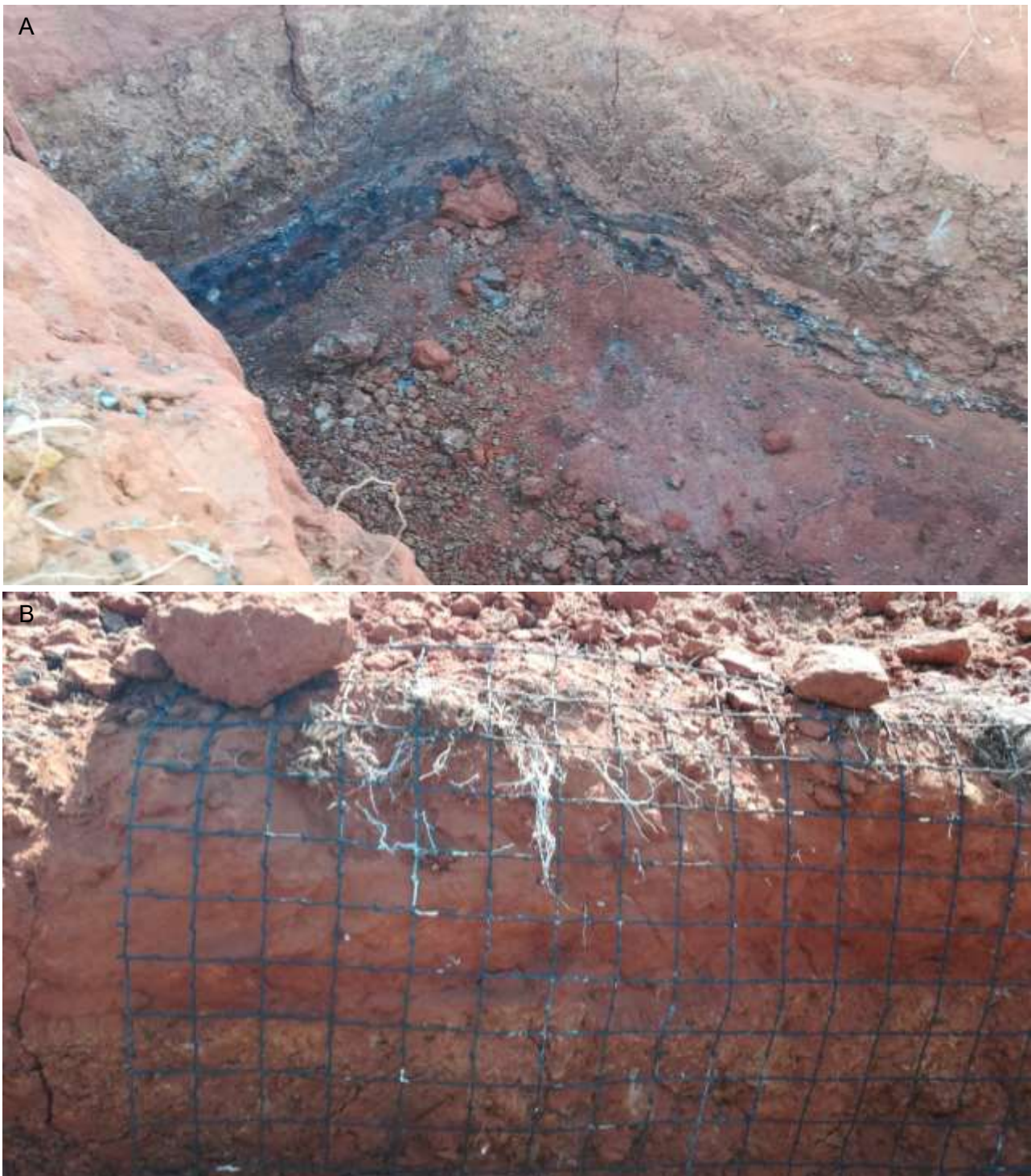
Figure 2.3: Vertical cracks through severely compacted layers at D2-1 (A) and, vertical and lateral cracks in severely compacted layers at D2-2 (B). Cracks can act as preferential flow paths for (nearly) saturated flows. Soil cover layers with high bulk density may not effectively function as water retention layer due to potential preferential flows through vertical and lateral cracks. Little water losses through plant transpiration will occur as no roots have penetrated and developed in the soil cover layers of D1-2 & 2-2 with high bulk density.
