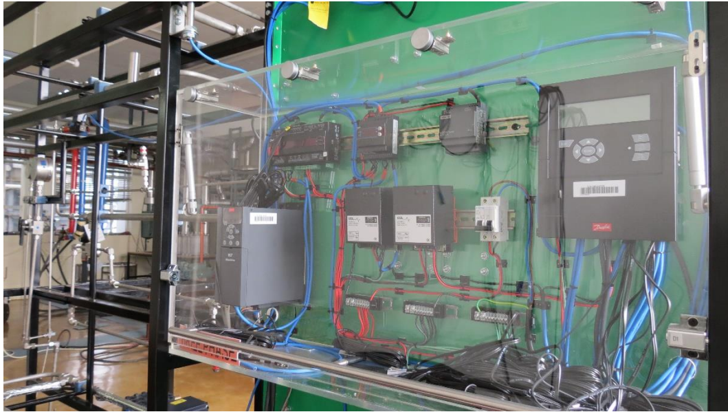
Figure 5.4 Photograph of Controller Box
