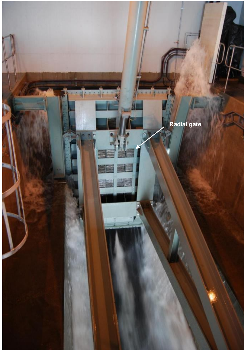
Photograph 16: Inside radial gate chamber
