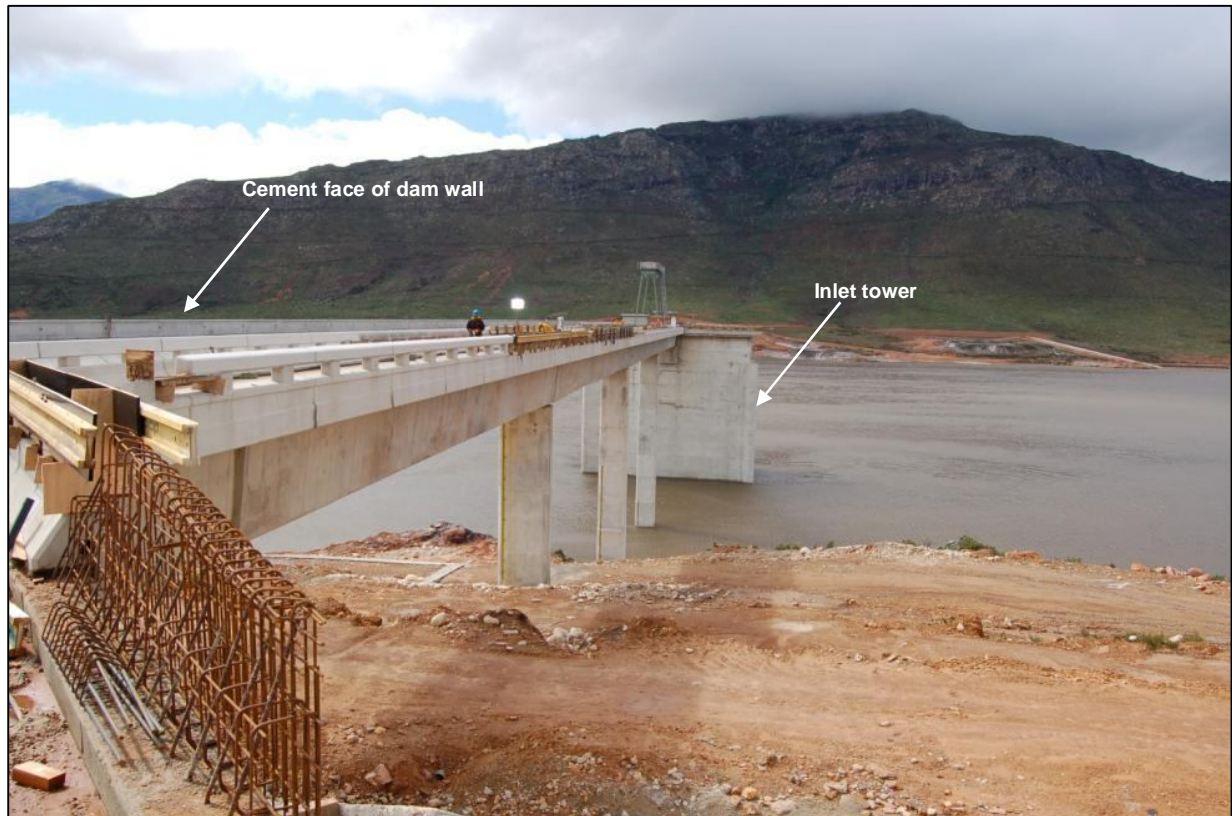
Photograph 19: Inlet tower (wet and dry well) and bridge to inlet tower under construction
