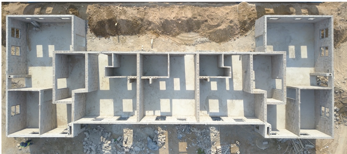
Figure 24. Picture of HDDS units taken from above with Drone
