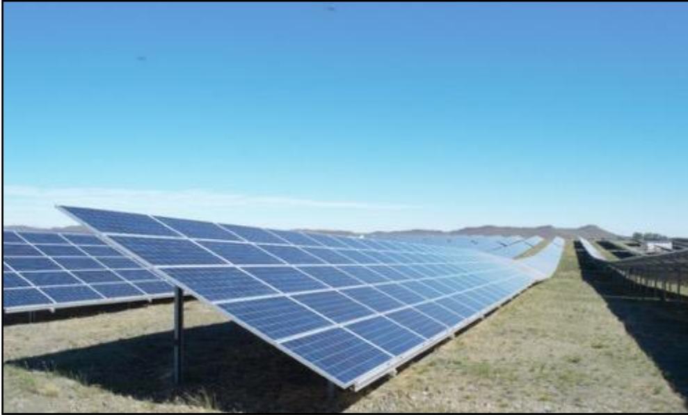
Figure 1.4: Solar panels on the De Aar Solar Power farm, April 2018
