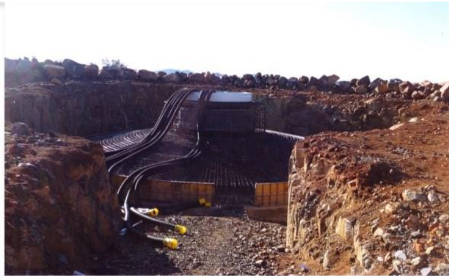
Appendix 14: Photographs taken by farmer during the construction phase of the wind farm
