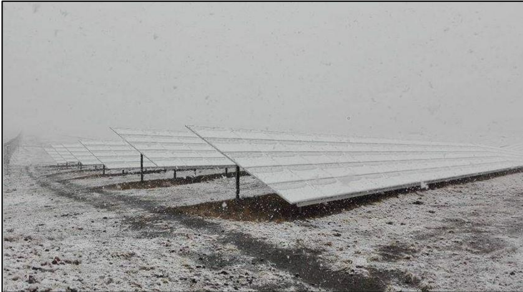
Figure 3.4 Snow on the solar panels from one of the IPP's in De Aar, 2018
