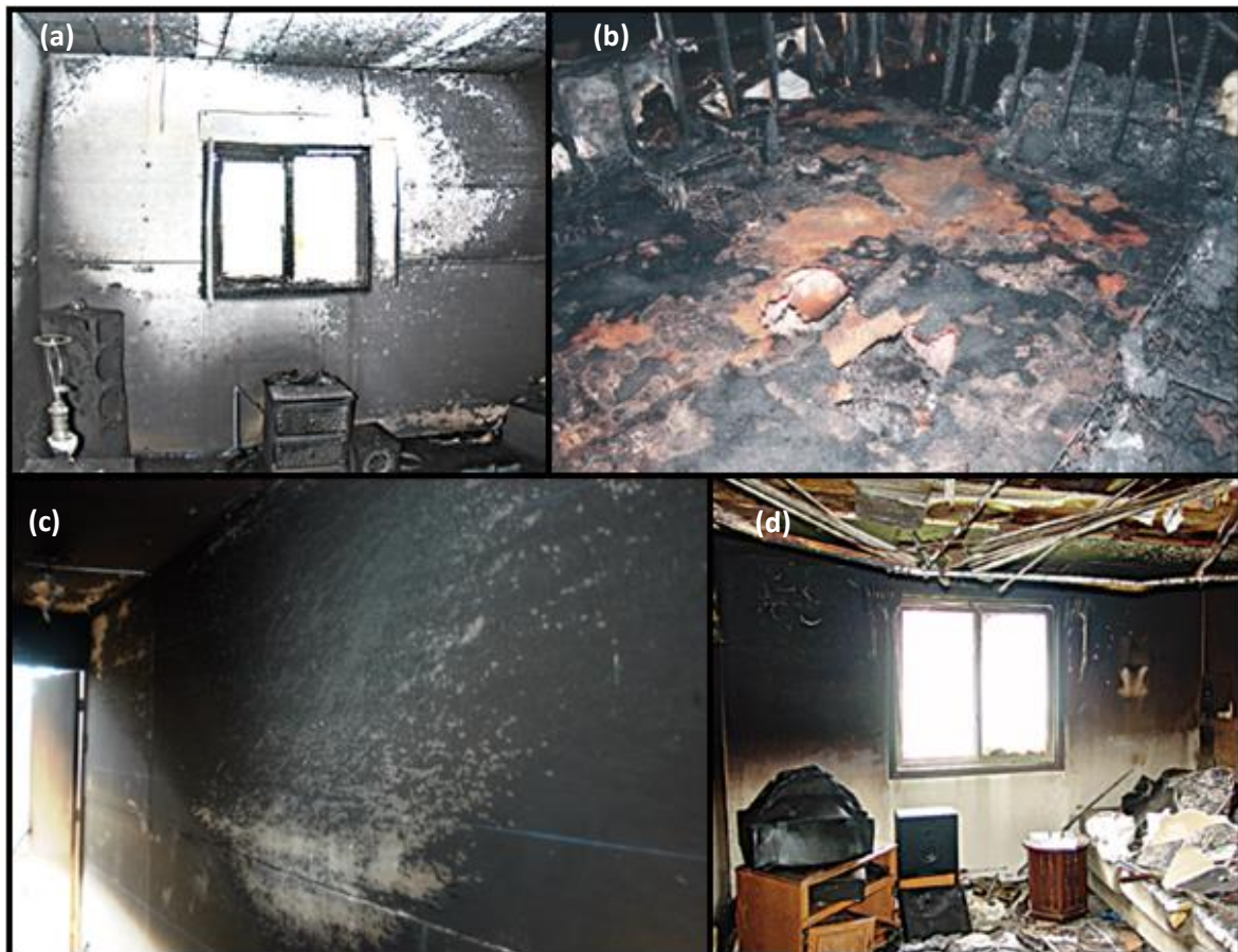
Fig. 2-7: Fire Patterns [59]. (a) Ventilation-Generated. (b) Full Room Involvement-Generated. (c) Suppression-Generated. (d) Hot Gas Layer-Generated.
