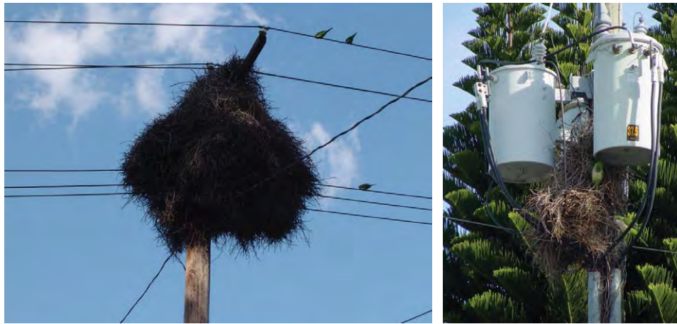
Fig. 10.6. Nesting Monk Parakeets on electrical infrastructures. (©Photographer: E.A. Tillman, courtesy of USDA/APHIS.)
