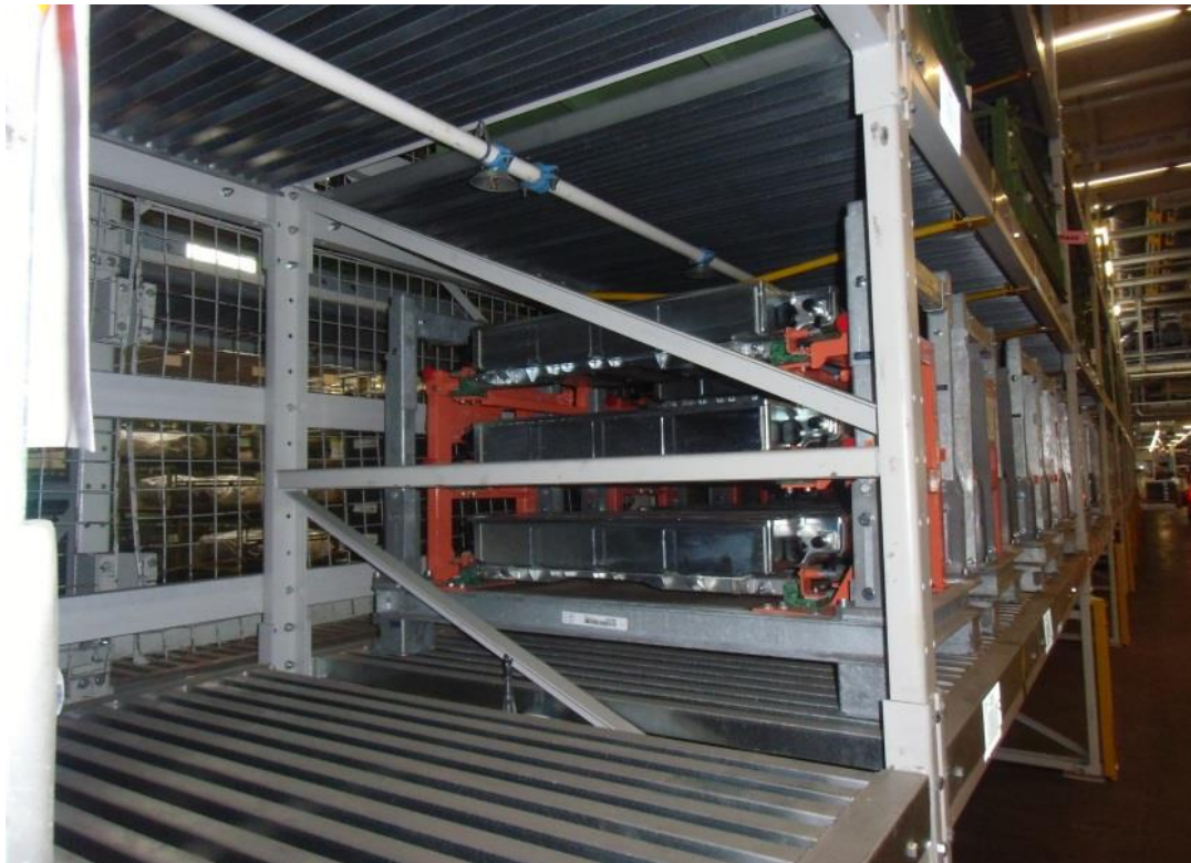
Figure 94: Sprinkler system in HV Battery warehouse section
