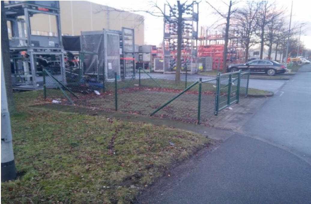
Figure 93: Dedicated emergency storage bay for damaged batteries
