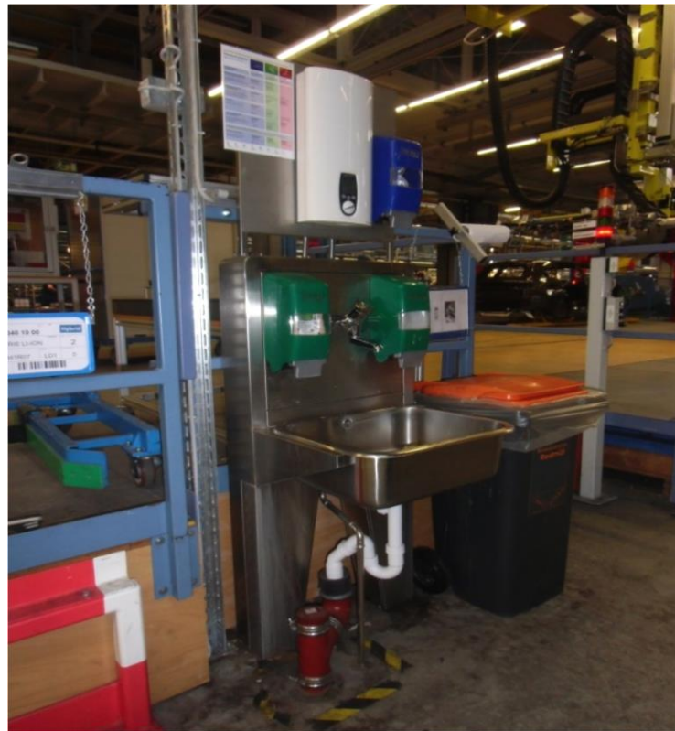
Figure 92: Hand and eye-wash station at Battery fitment station
