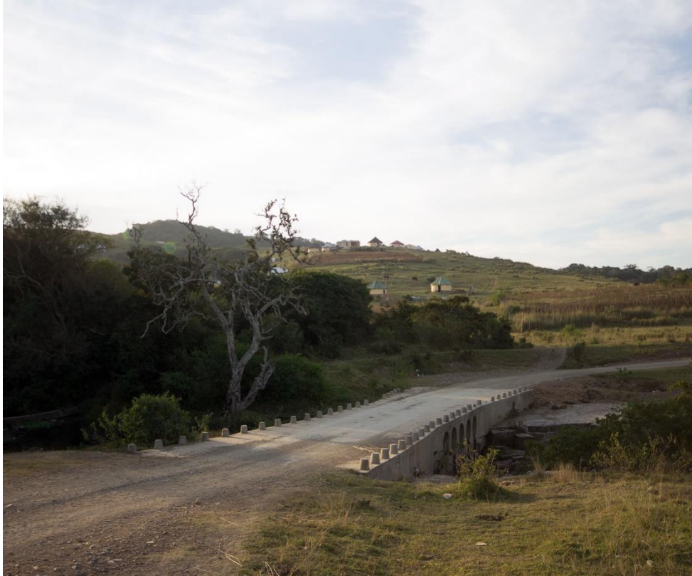
Figure 5.2: Photo of the bridge that leads into Community A. Once the bridge is flooded the community gets cut off from the other communities.
