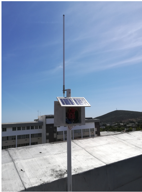
Figure 5.23: An assembled WSN node, with the antenna and solar panels attached.
