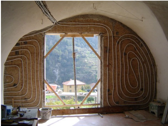
Photo 4.17. Heating system (Sources: Torri website).
