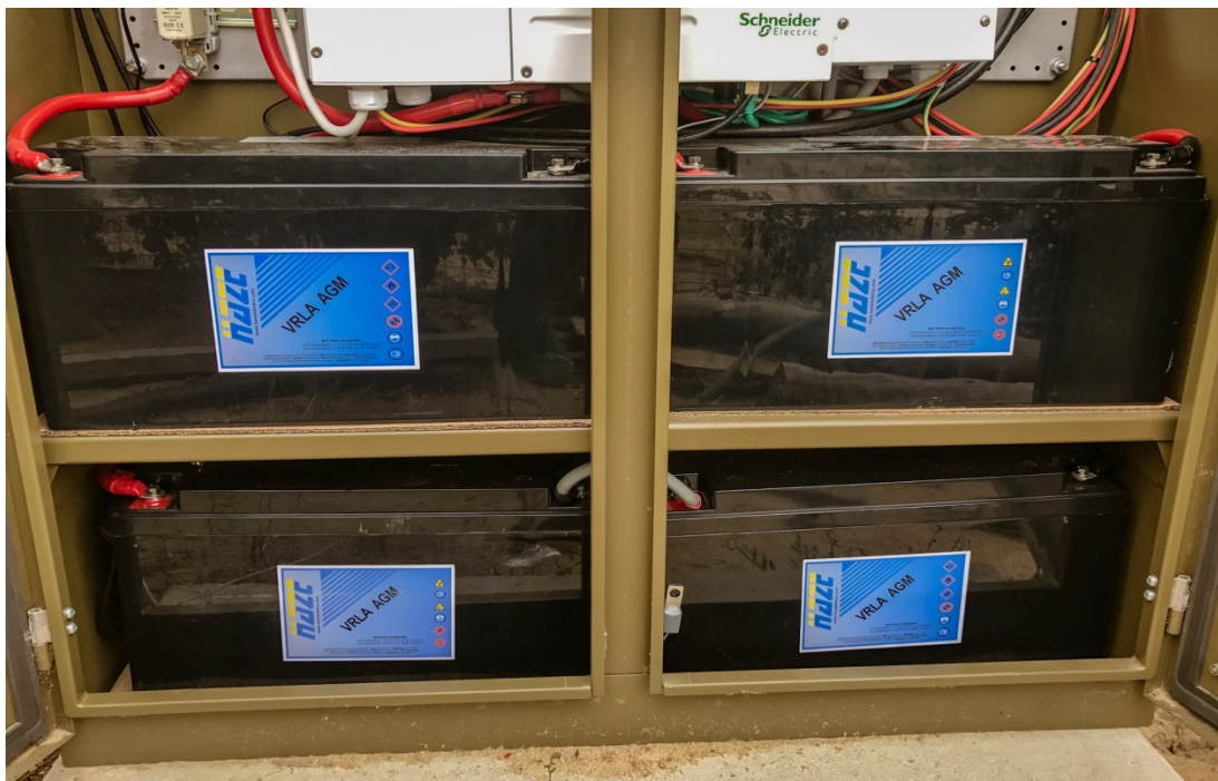
Photo 4.30. Batteries (Source: Sharné Bloem).
