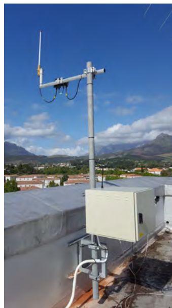
(b) Sigfox base station
