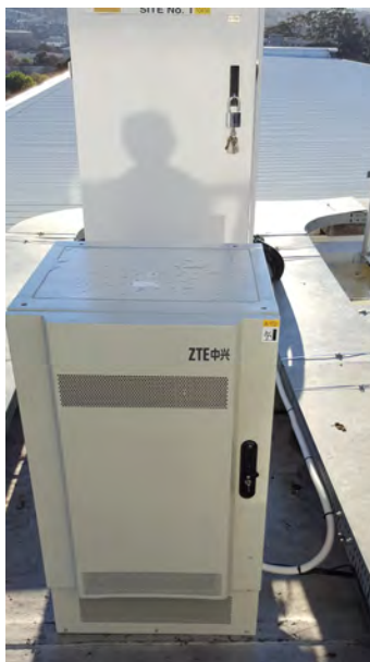
(a) NB-IoT base station
