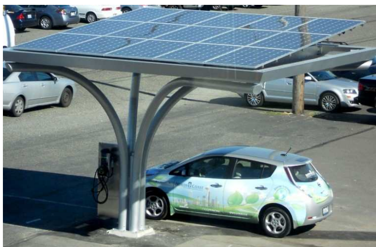
Figure 2.10: Solar-powered Electric Car Charger – City of Cape Town
