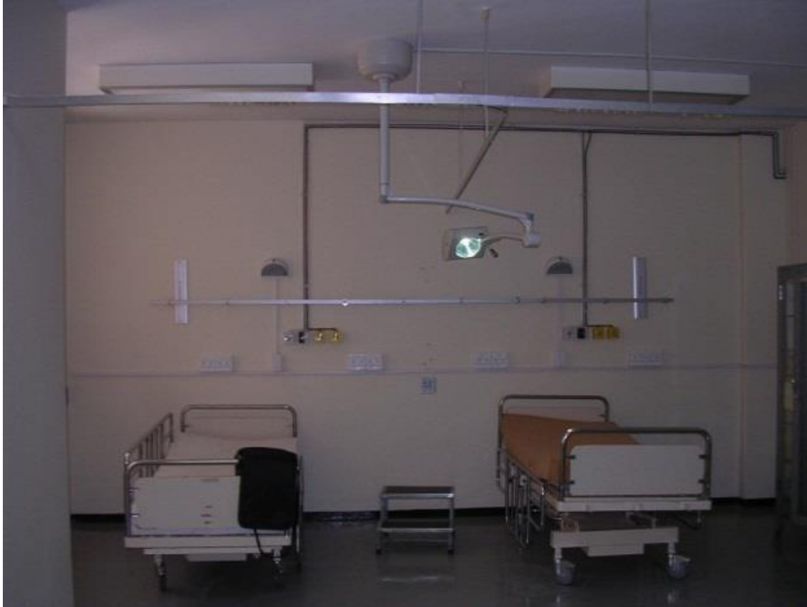
Photo 2: Permanent infrastructure fixtures and wall bedside layout
