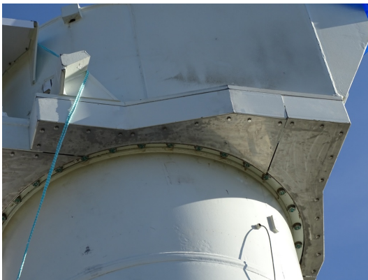
(a) Covers prohibiting access to the shoe-slip ring assembly.
