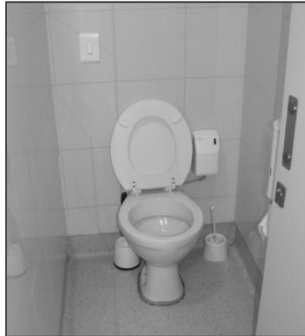
Figure 3.12: Second Movement toilet installed at the green s'cool at Old Mutual Park , indicating the flushing mechanism (top left).
