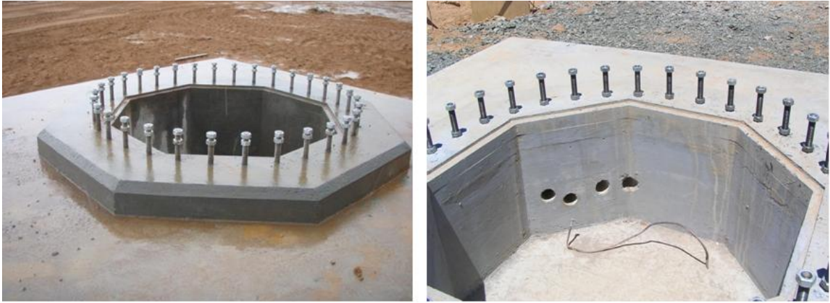
Figure 6.2: Photographs of the foundation showing the foundation bolts on the concrete lip on the left, and the space provided for cable entry on the right.
