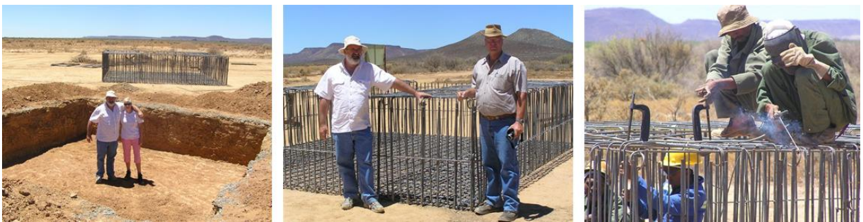
Figure 6.30: Photographs f.l.t.r. The foundation excavation for one of the KAT-7 antennas with the steel reinforcing to be used in the background; The steel reinforcing for one of the structure foundations; Welding of foundation steel reinforcing elements to improve resistance to earth.
