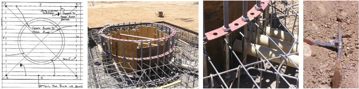
Figure 6.31: F.l.t.r Early design sketch of the earth electrode layout; The pedestal mounting foundation bolts connected to the reinforcing; Earth electrode connected to the foundation ring with a bolted lug; Exo-thermic welding connection for the earth electrode conductors.
