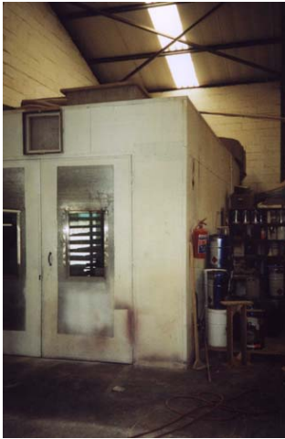
(a) Top Coat Spray-booth
