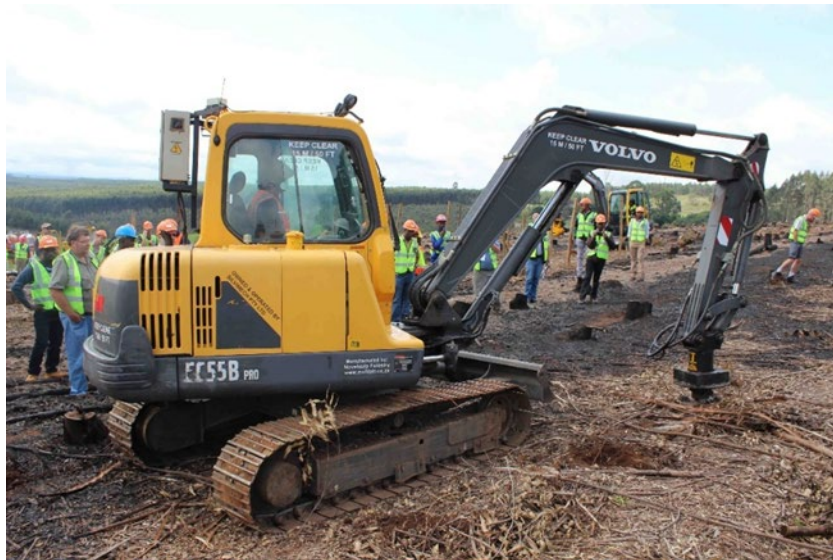
Figure 2.1: Volvo compact excavator, (EC55B) fitted with the, Mpat pitting head and control system (Chapman, 2015).
