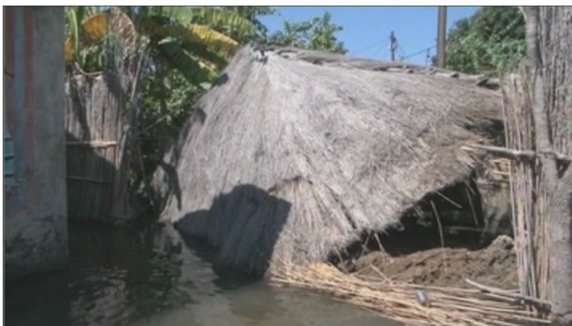
Figure 5.14: A traditional hut that has collapsed due to excessive water of Efundja (Image used with kind permission of Namibia Broadcasting Cooperation of Namibia).
