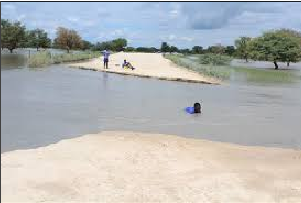
Figure 6.4: An example of a road that has been washed away during the rainy season
