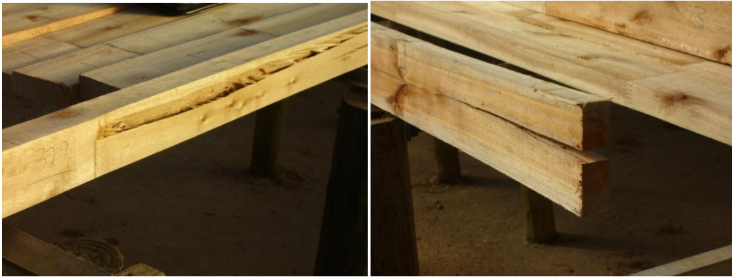
Figure 14: Severe surface check (left) and end-split (right).
