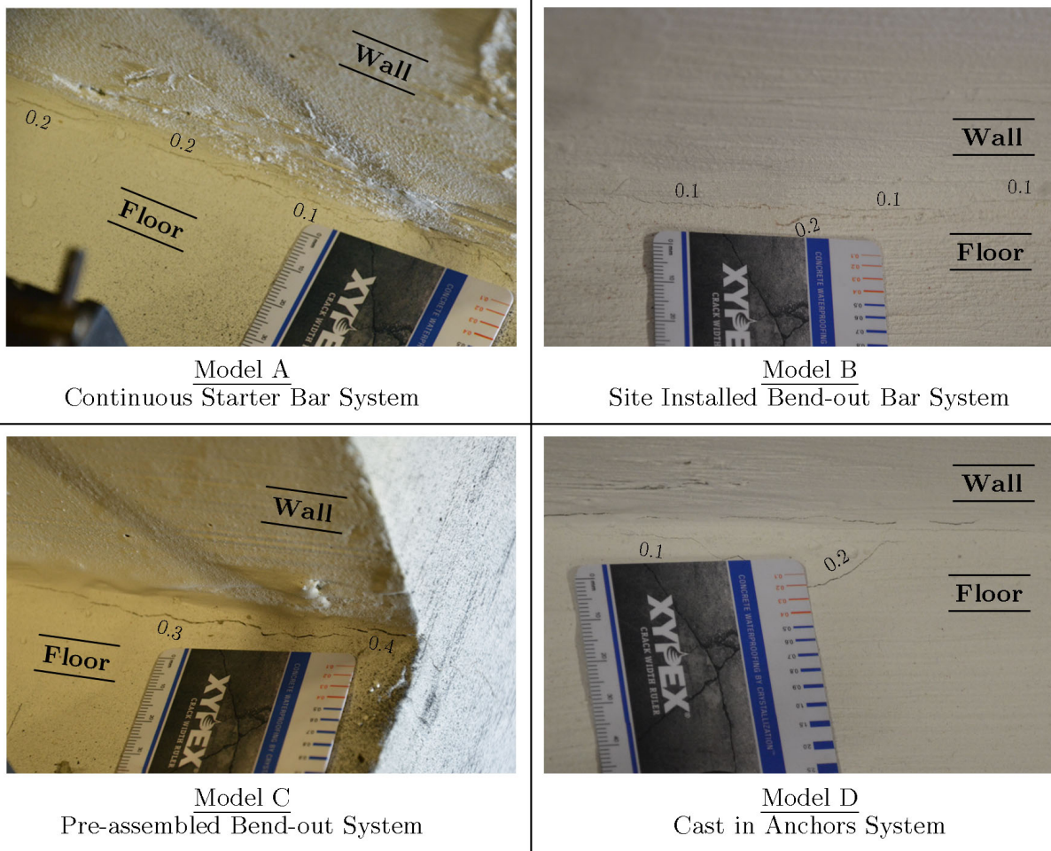
Figure 4.2: Cracks at Stage 1 - Top of Floor
