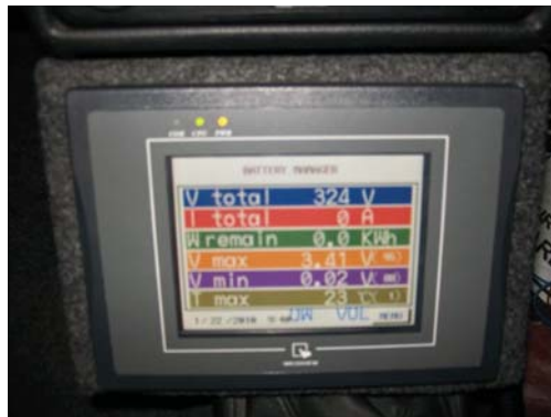
Figure 3.5: Display unit of the battery management system.
